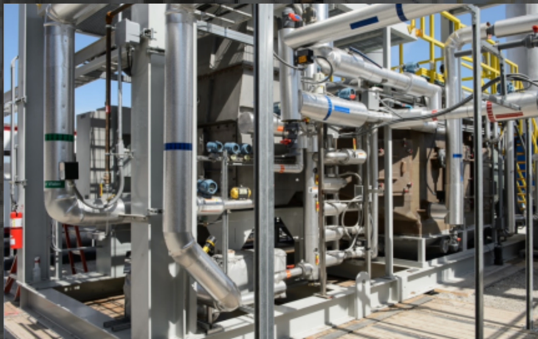
Figure 3. A side view of the Heartland Concentrator at Power Plant.
