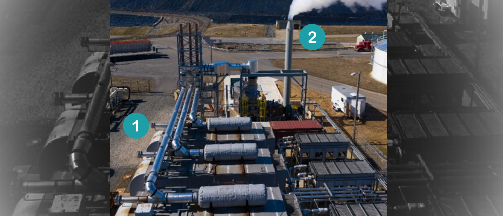
Figure 3. (1) Hot generator exhaust gas is ducted together to provide thermal energy for evaporation in the Heartland Concentrator™ (2)
