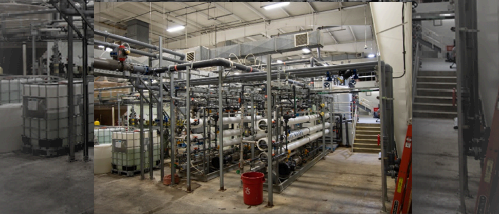
Figure 2. Concentrated Leachate from the RO Plant requires treatment
