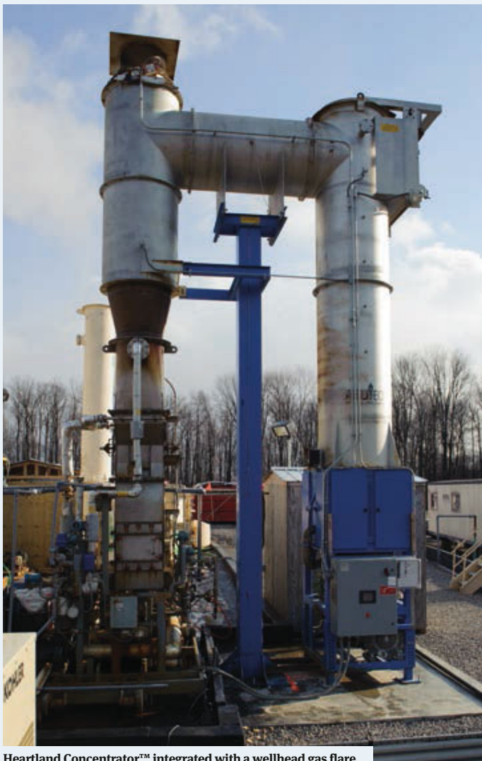
Heartland Concentrator™ integrated with a wellhead gas flare.
