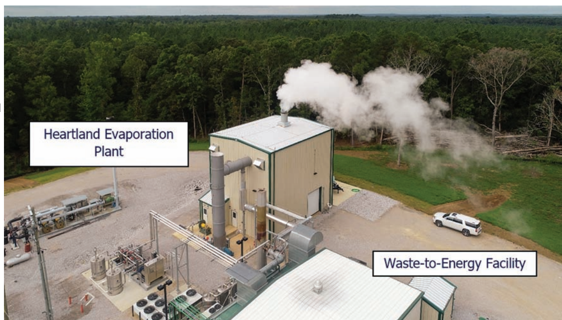
Figure 1 Overhead view of the 25,000 gpd Hybrid CoVAP™ Leachate Evaporation Facility.
