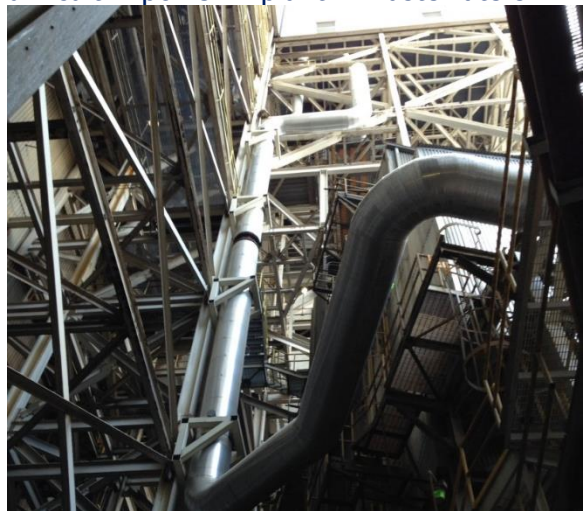
Figure 3. Flue gas ductwork from Bowen's Unit 3 feeding the Heartland Concentrator.
